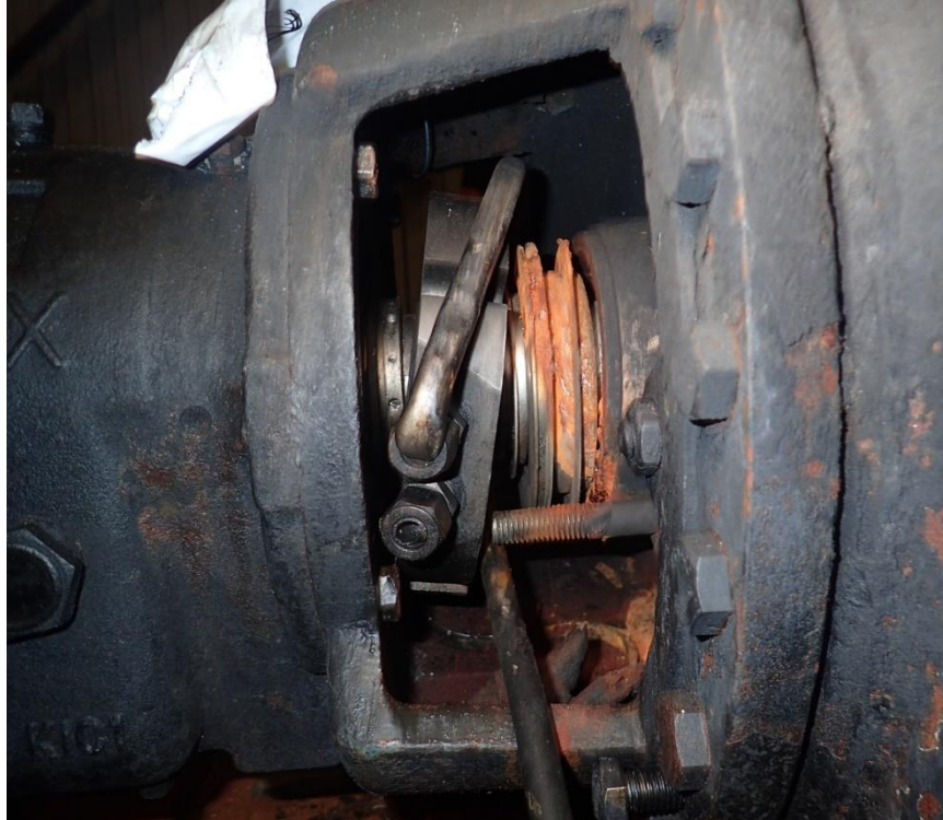
Fig. 3 – Seal Chamber Closeup, Alternate Angle
